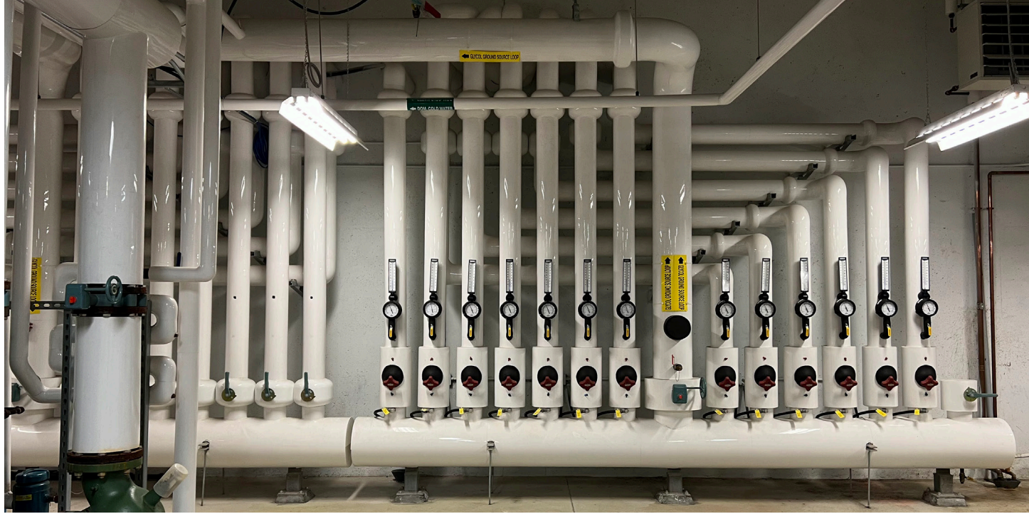
Geothermal distribution pipes in the mechanical room of the Instructional Centre
